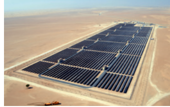
Phase 1 Mohammed bin Rashid al Maktoum Solar Park Seih Al Dahal, Dubai
